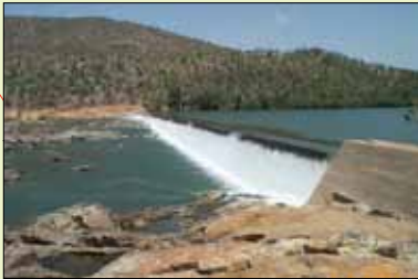
GORGE WEIR - Capacity 9,460 Megalitres
