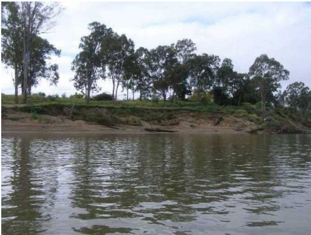
Photograph 9 Eroded River Bank, Fig Tree Pocket.
