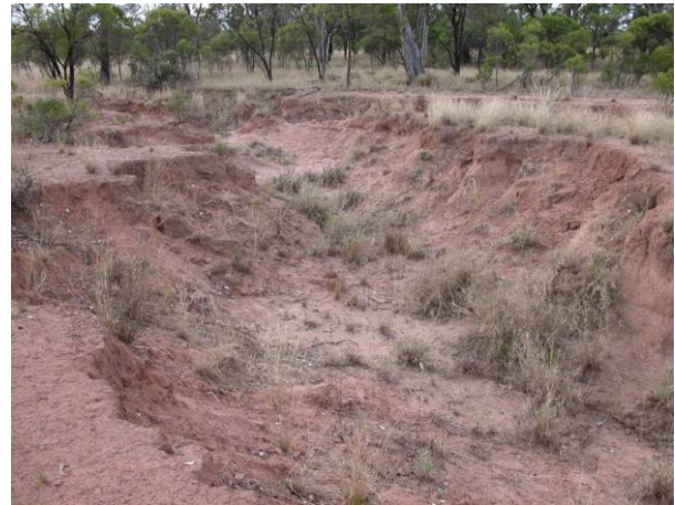
Erosion gullies on the edge of the main channel of Wallam Creek have been targeted for repair.
